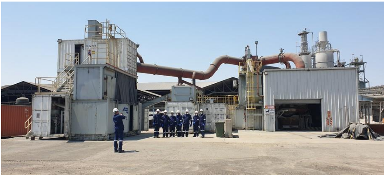
DST’s GlassLock arsenic stabilization facility in Namibia. Credit: Dundee Sustainable Technologies
